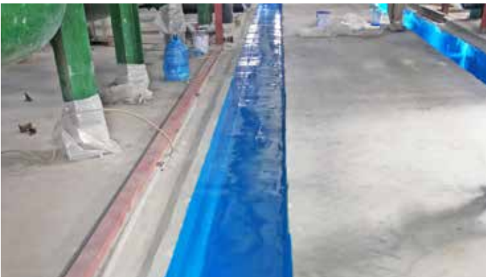
The primer coat of ChemLINE® (blue color) is also applied into pit channels (trenching).
