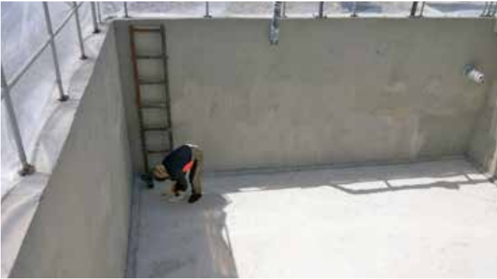
The concrete secondary containment surface is first cleaned and prepared for the coating application.
