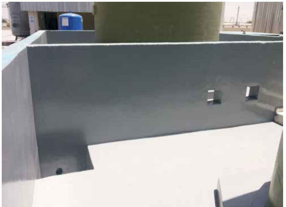
Secondary containment area lined with ChemLine® coating.
