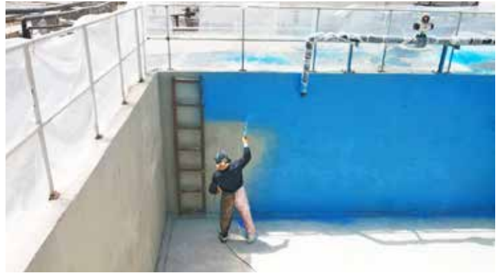
The primer coat of ChemLINE® (blue color) is sprayed onto the concrete secondary containment pit.
