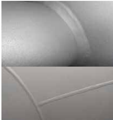
Proper profile of carbon steel surface with all welds and seams inspected
