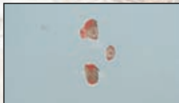
2. Close-up of damage area to repair.
